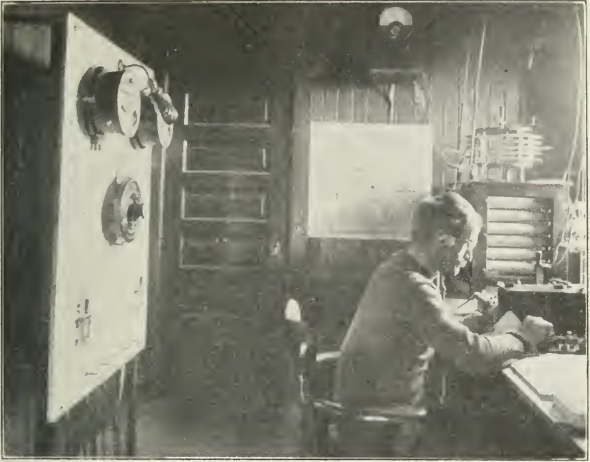
THE INTERIOR OF A HIGH POWER STATION
